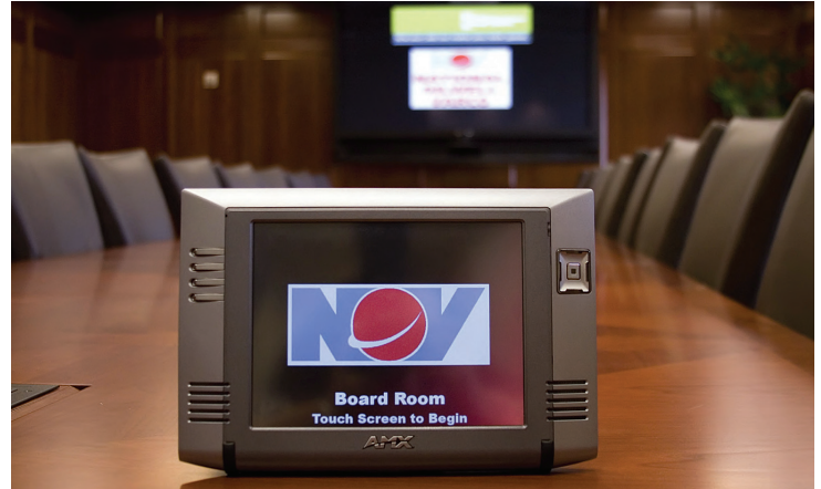
Custom AMX programming made it so that the cascading inserts in the boardroom's table open in sequence at the same time the plasmas are lowering from the ceiling.
